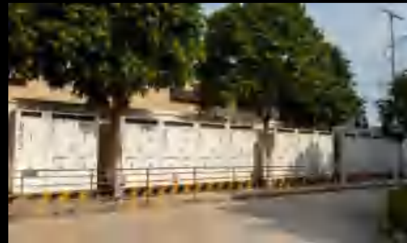
Guangdong Huizhou user-side energy storage project
