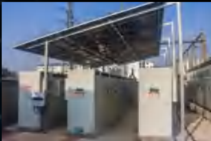
Hunan Yongzhou grid side energy storage project
