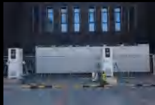
Beijing Yizhuang Development Zone storage and charge integrated project
