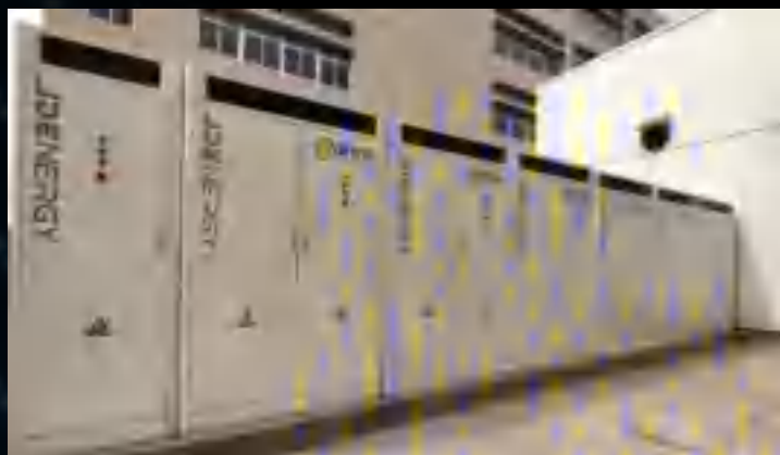
Guangzhou Panyu user-side energy storage project
