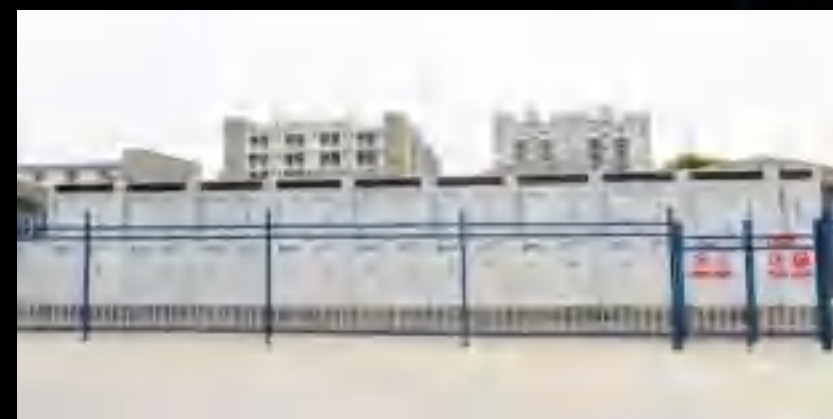
Guangdong Dongguan user side energy storage project
