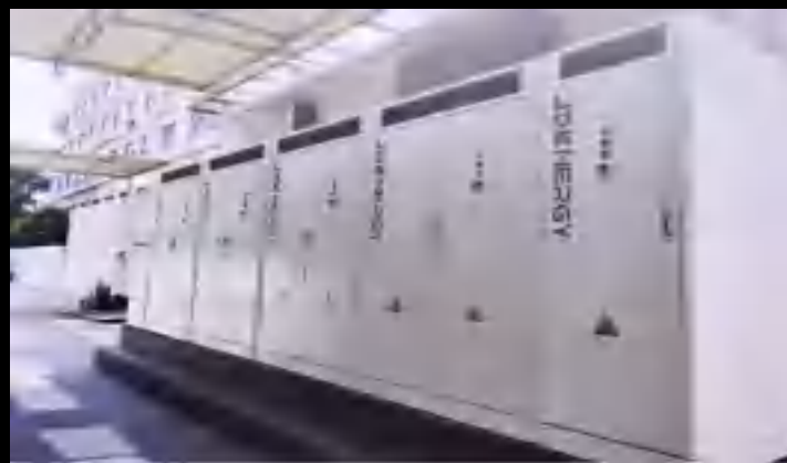
Zhejiang Yiwu user-side energy storage project
