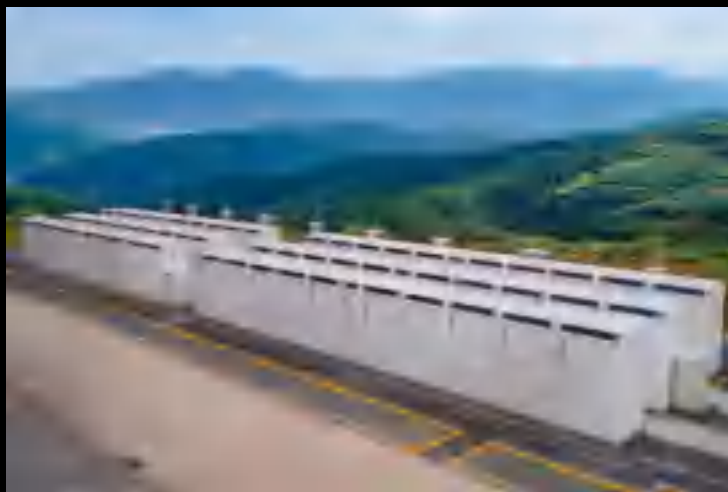
Chongqing Changshou 10MWh energy storage project
