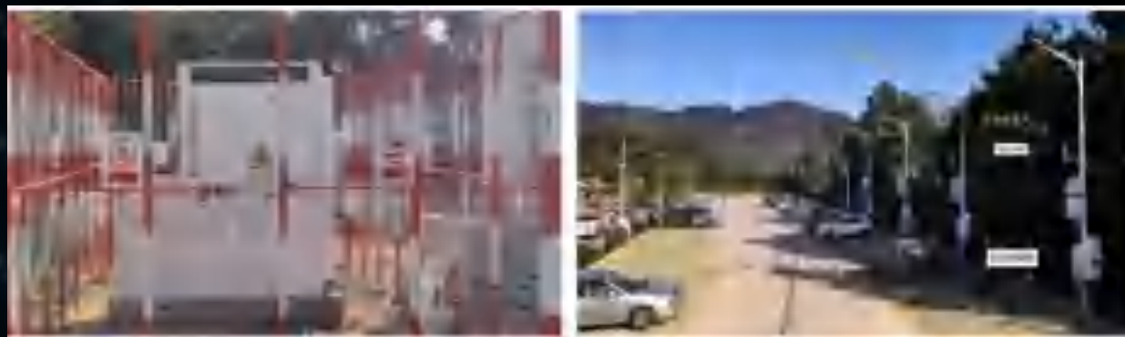
Qingyuan beautiful village energy storage project
