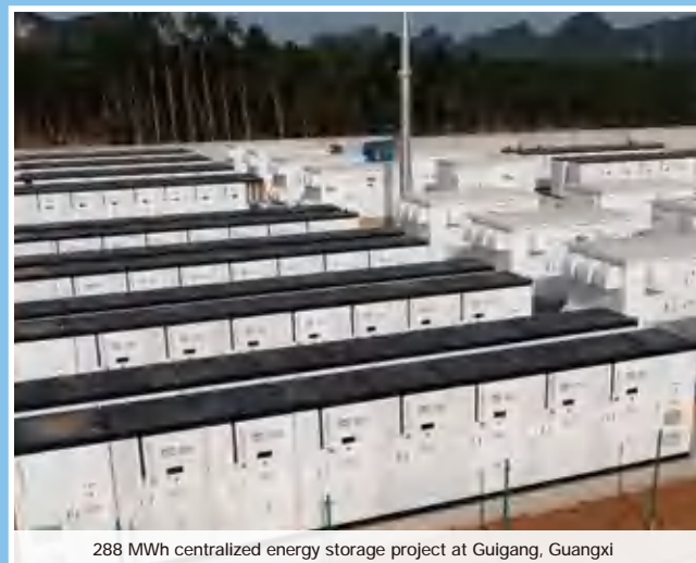
288 MWh centralized energy storage project at Guigang, Guangxi
