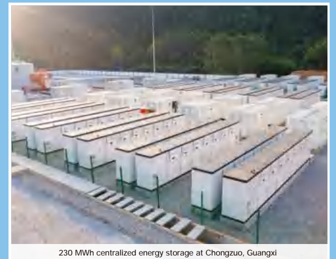
230 MWh centralized energy storage at Chongzuo, Guangxi
