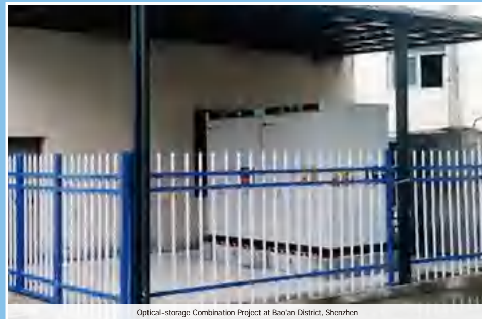
Optical-storage Combination Project at Bao'an District, Shenzhen
