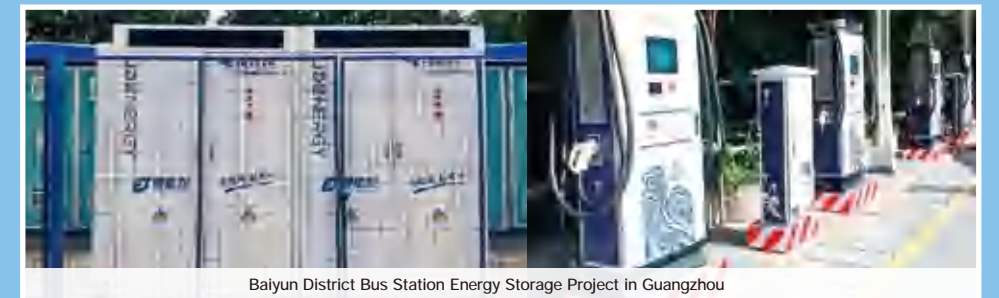
Baiyun District Bus Station Energy Storage Project in Guangzhou
