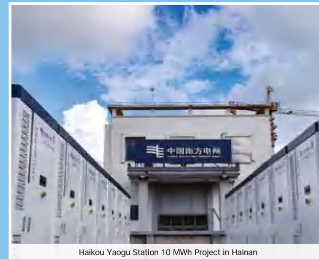
Haikou Yaogu Station 10 MWh Project in Hainan
