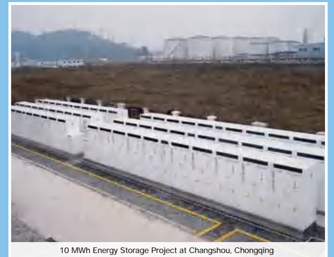
10 MWh Energy Storage Project at Changshou, Chongqing
