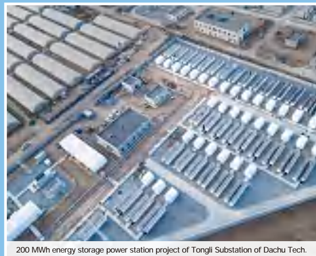
200 MWh energy storage power station project of Tongli Substation of Dachu Tech.
