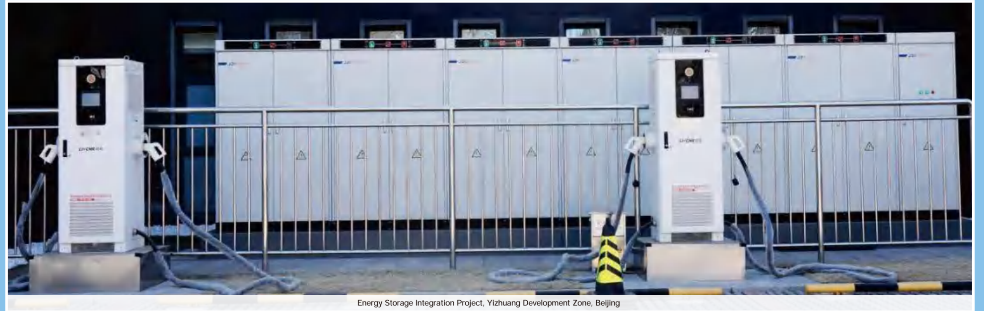
Energy Storage Integration Project, Yizhuang Development Zone, Beijing
